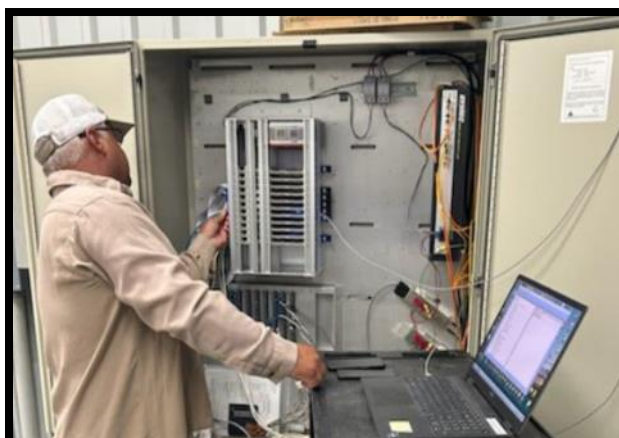
SCADA Technician Programming the New RTU at Palacios.
