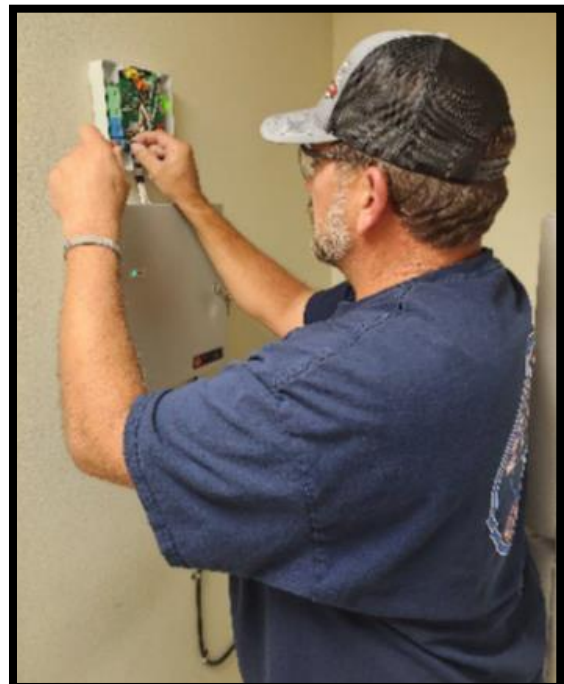
Axis Door Access Control.
